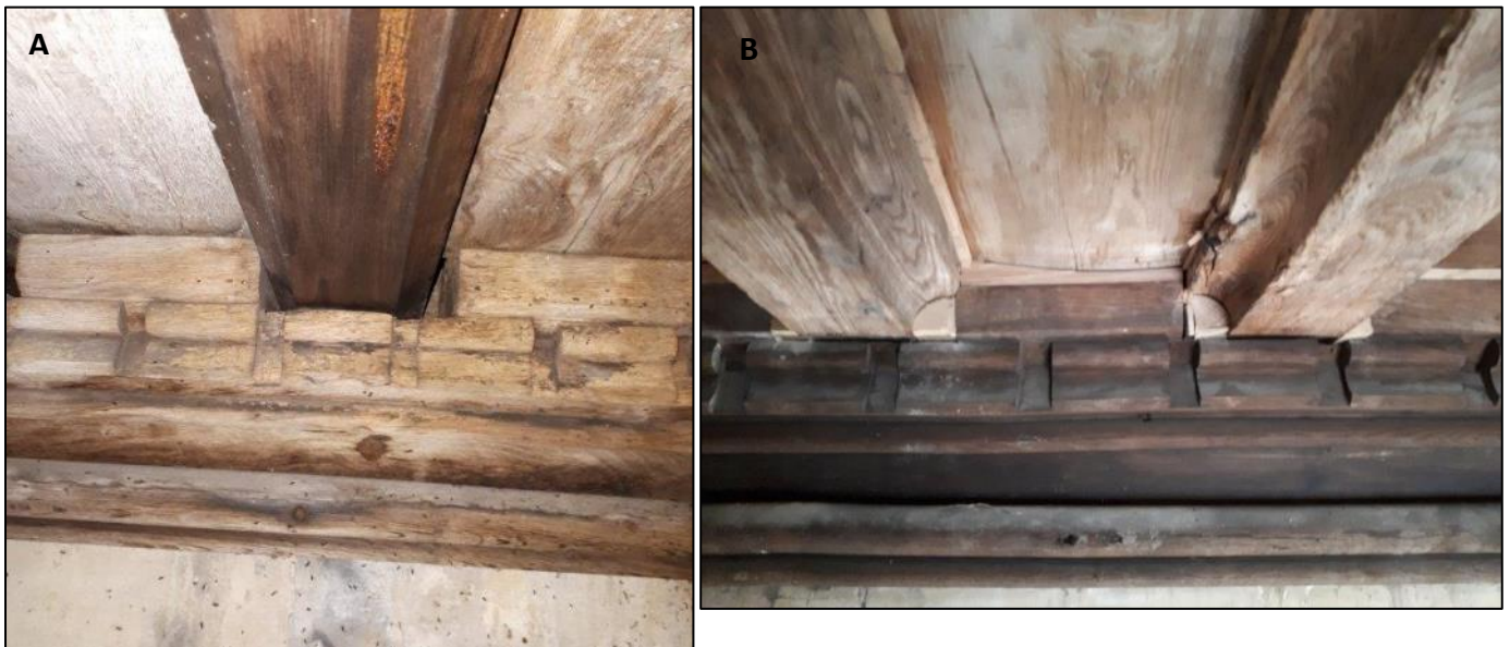
Figure 4: Photo A shows the gaps in the timber above the servery of Holy Trinity, Tattershall, used by soprano pipistrelles to roost. Photo B shows the closing of roosting opportunities above the servery. © BJ Collins Ltd.
