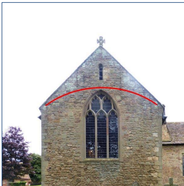
Figure 26: There is an enclosed void above the timbered barrelled ceiling in the chancel (indicated by red line). The meshing of the lancet aperture has been opened to provide a potential alternative roost site for the colony of Natterer's bats currently using the church interior.
