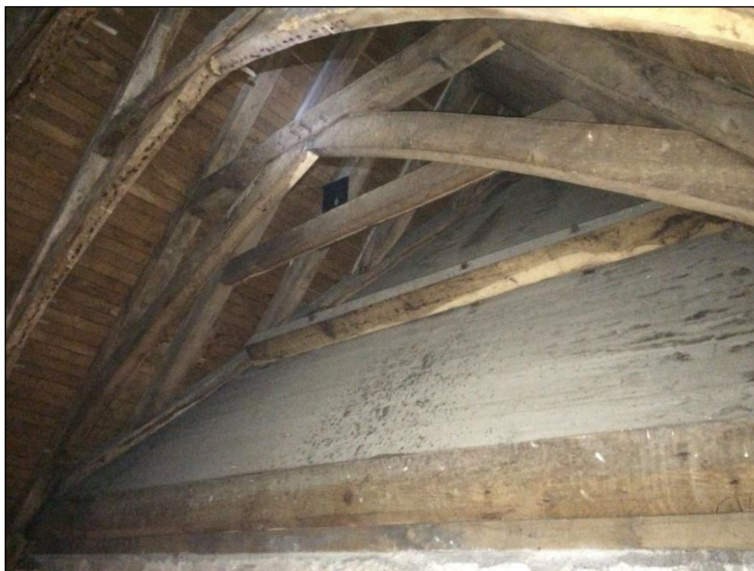
Figure 5: Bat droppings and urine staining in the roof void of St Mary the Virgin, Pembridge, Herefordshire.
