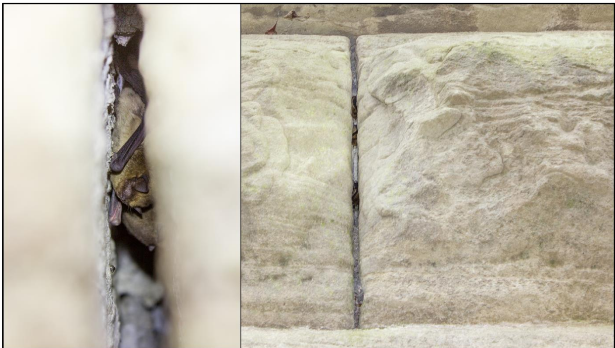
Figures 2 and 3: Pipistrellus bats roosting in viaduct crevices. Close view on left, zoomed out on right.
